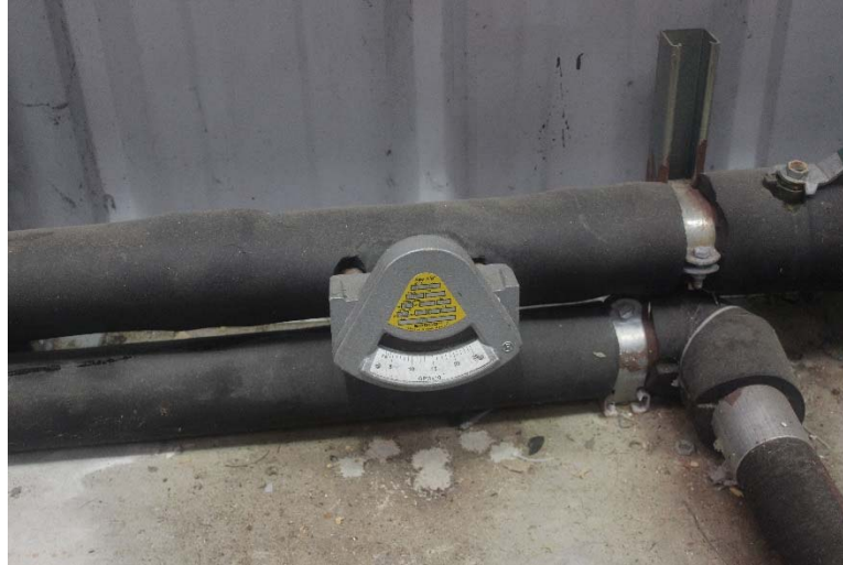
Figure 4 – Flow meter (behind chiller)
