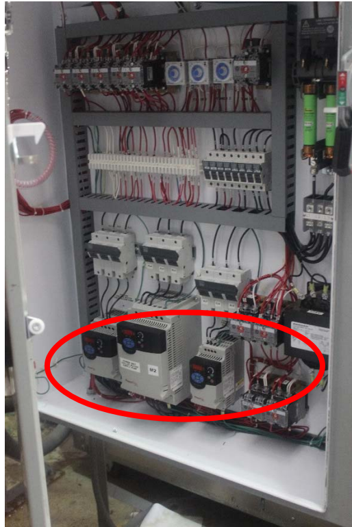
Figure 2 – Chiller control panel interior
