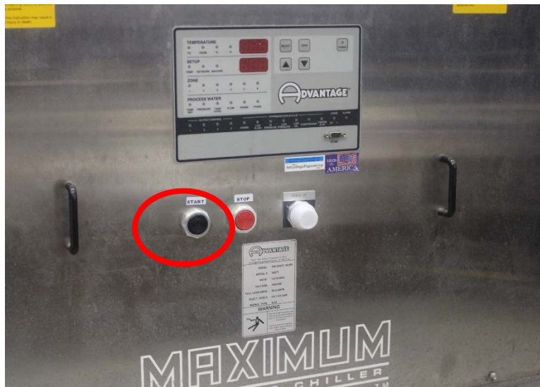
Figure 3 – Chiller front panel
