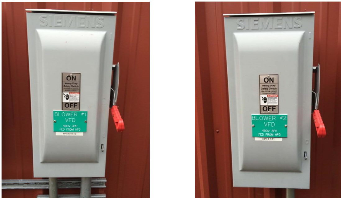
Figure 3 – Variable Frequency Drive 1 & 2 Electrical Breaker Boxes
