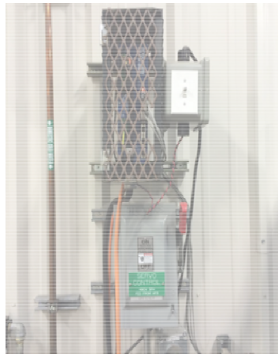
Figure 7 – Servo motor breaker box and switch
